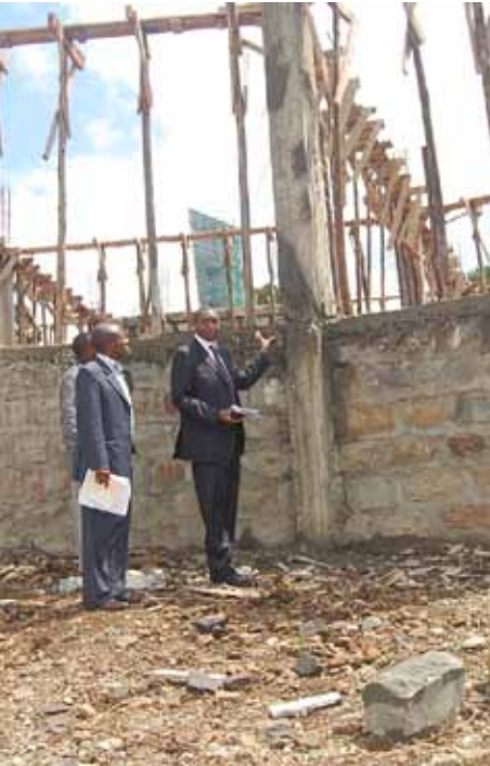
KNLS Director (right) with the project manager inspect the construction of Narok library in June 2011
